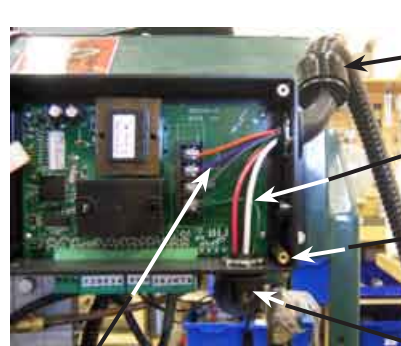
Motor Control Wires
